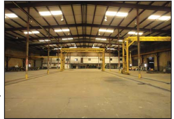
Phase 1 Bridge Cranes
